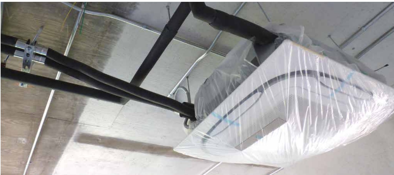
Insulation from Branch Controller to the ceiling cassette
